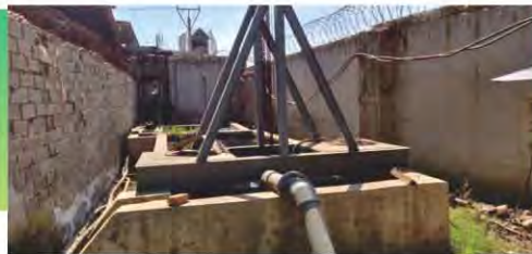
Wastewater recycling pool
