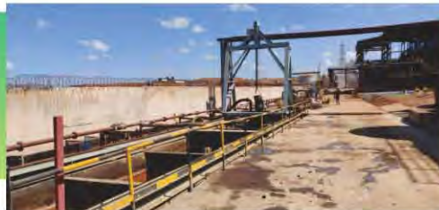
Sedimentation tank Level-5
